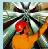
Tunnel laid GIL
