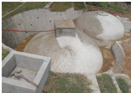
Fixed dome bio-gas system
