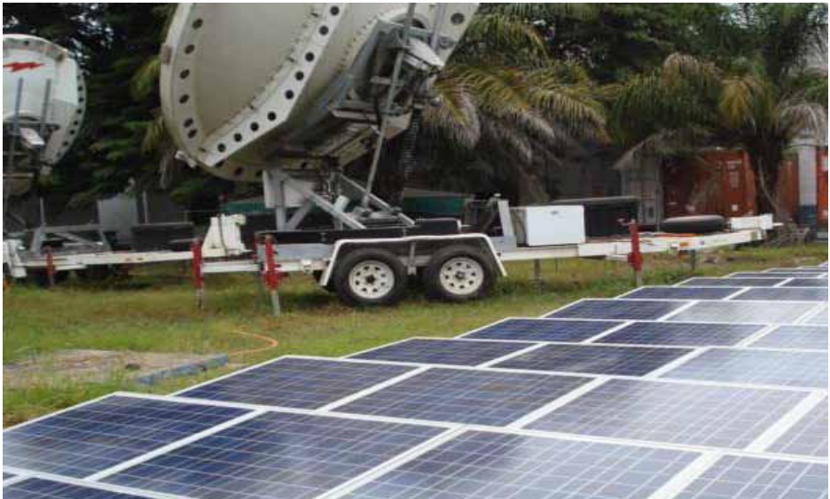
Solar Power Arrays at MONUC HQ
