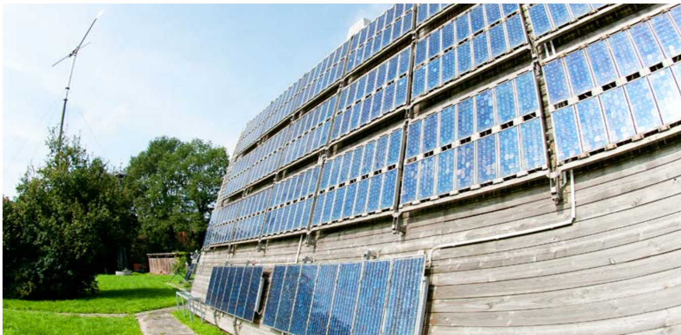
„The trajectory of research on renewable energies“. The plans for the self-sufficient Energy Lab – with its photovoltaic systems pictured here – were developed in the 1970s.
